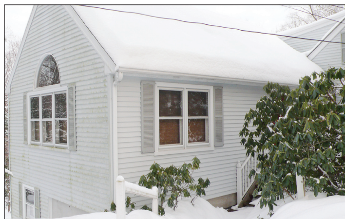
Before Photo In the 25-year-old addition, the double-paned windows will be retained, while the rest of the structure will be modified to improve building energy efficiency, moisture-barrier performance and architectural appeal.
