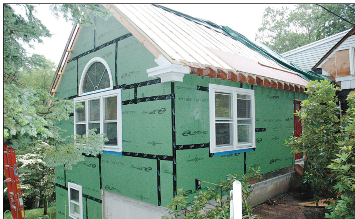
Construction Photo Rigid foam insulation has been applied to the side walls with ZipWall sheathing, more than doubling the wall insulation R-value. All connections have been taped and foamed to minimize air infiltration. Windows have been reset, sealed, flashed and trimmed with low-maintenance PVC. Work is underway on the roof, with the application of rigid foam insulation complete. Final side wall will be pre-finished white cedar shingles.
